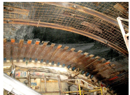
Rock mass failure 2007
